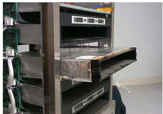
Fig. 17. Slide malfunctioning slot from cabinet.
