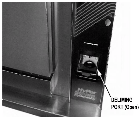
The De-Liming Port is at the Bottom of the Control Panel.
