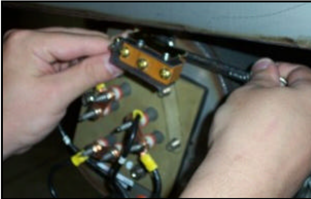
Tightening the brass fitting.
